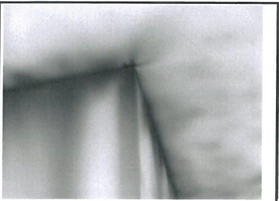
More air leakage/wall washing of air from attic
